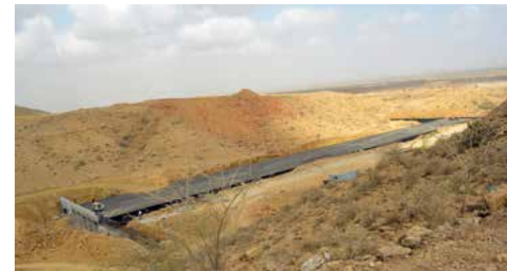
A road under construction in Gadap Town, Karachi, February 2016. Photograph by Zahra Malkani. Image courtesy: Zahra Malkani.
