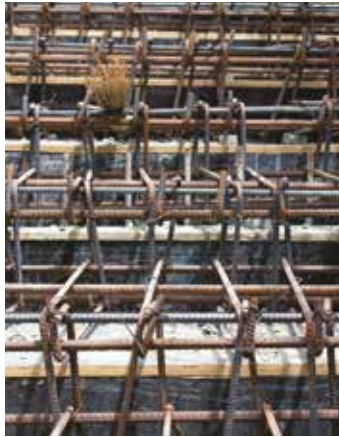
Top Left: Space No.1 – Rusted steel, bent to provide shape to the staircase. Photo by author
