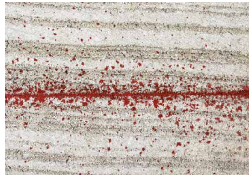
Space No.1 – Splashes of red oxide markings. Photo by author
