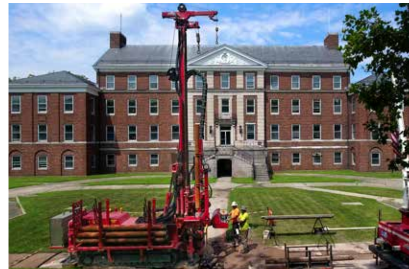
Rotosonic drill near historic hospital extracting continuous core down to 125ft.—through glacial till, original 19th century seawall, to bedrock.
